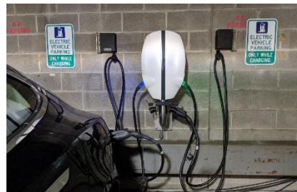
Electric Vehicle Charging Stations installed at our Rittenhouse Hotel, Philadelphia, PA
