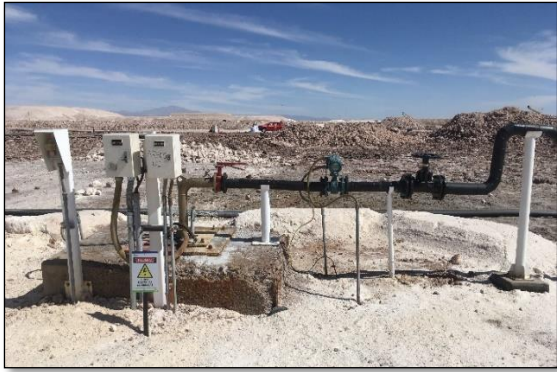
a) Brine production wells with surface equipment
