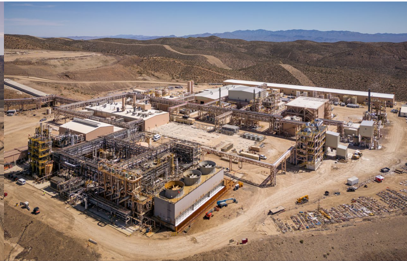
Midstream Separation & Refining
