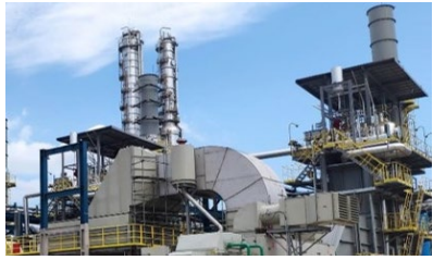
1st Low Emissions Gas Turbines Running on Hydrogen Blend
