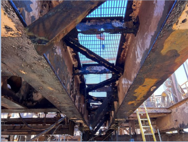
Collapsing Structures and deteriorated CIL tanks
