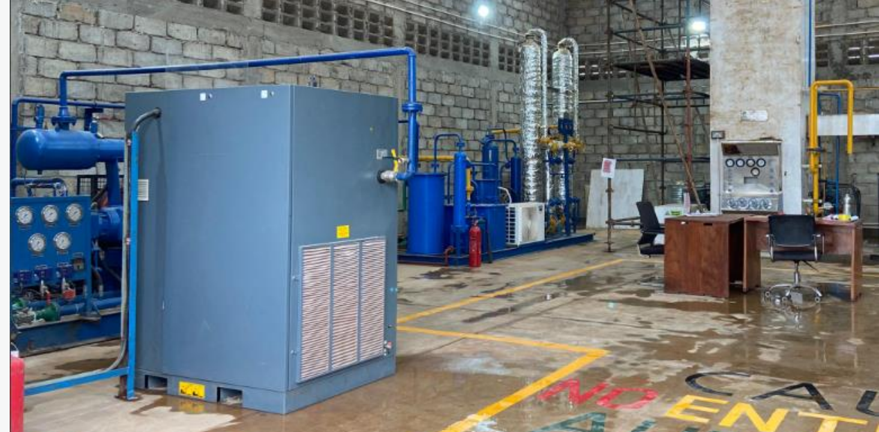
Gas production facility
