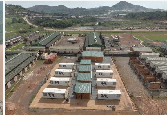
Additional battery storage containers
