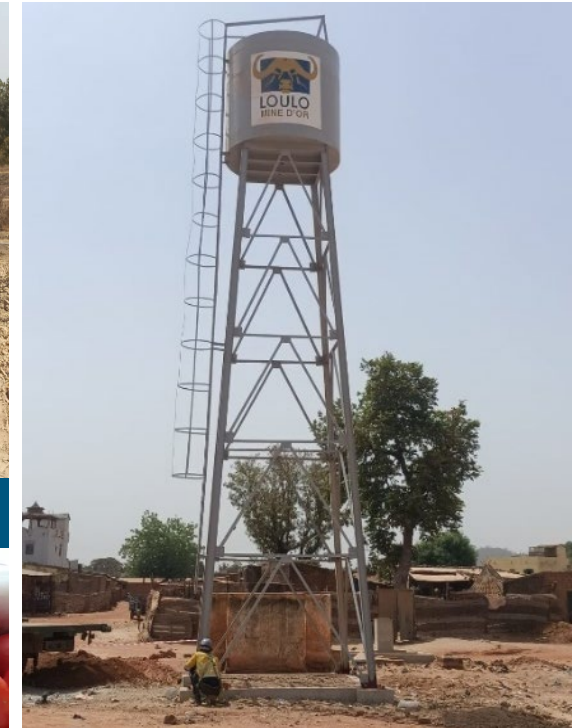
Water supply system built in Loulo village
