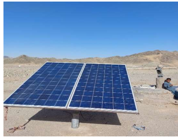
Solar Panels at Darband Chah Settlement
